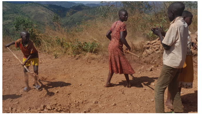
Children all joined to get the place for church building ready for construction.
