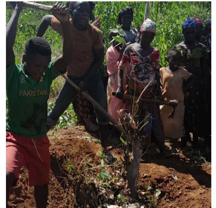
Children could not stay but joined the adults in uprooting trees for construction to begin.
